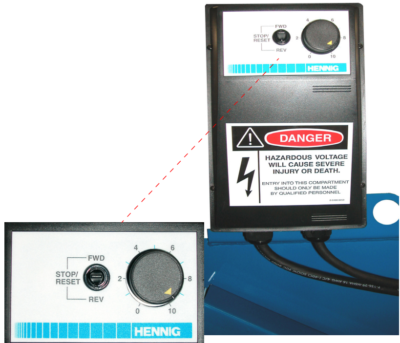
Figure 3-18: Control Operating Positions
